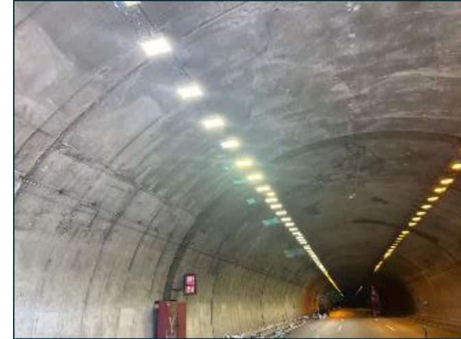
Selçukgazi Tunnel LED Transition
