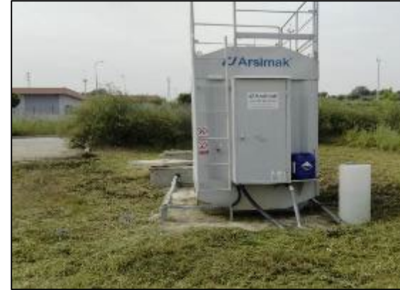
Waste Water Plant in O&M Center
